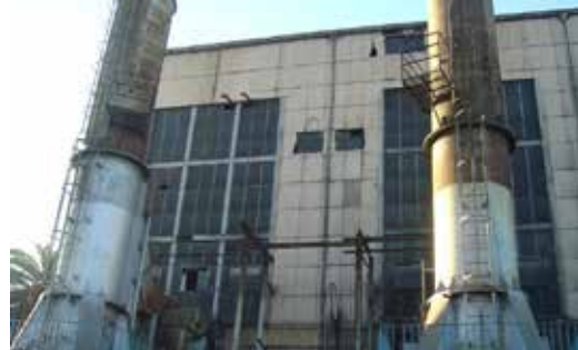
Buhar Santrali / Steam Power Plant (Uğursal, 2011)
